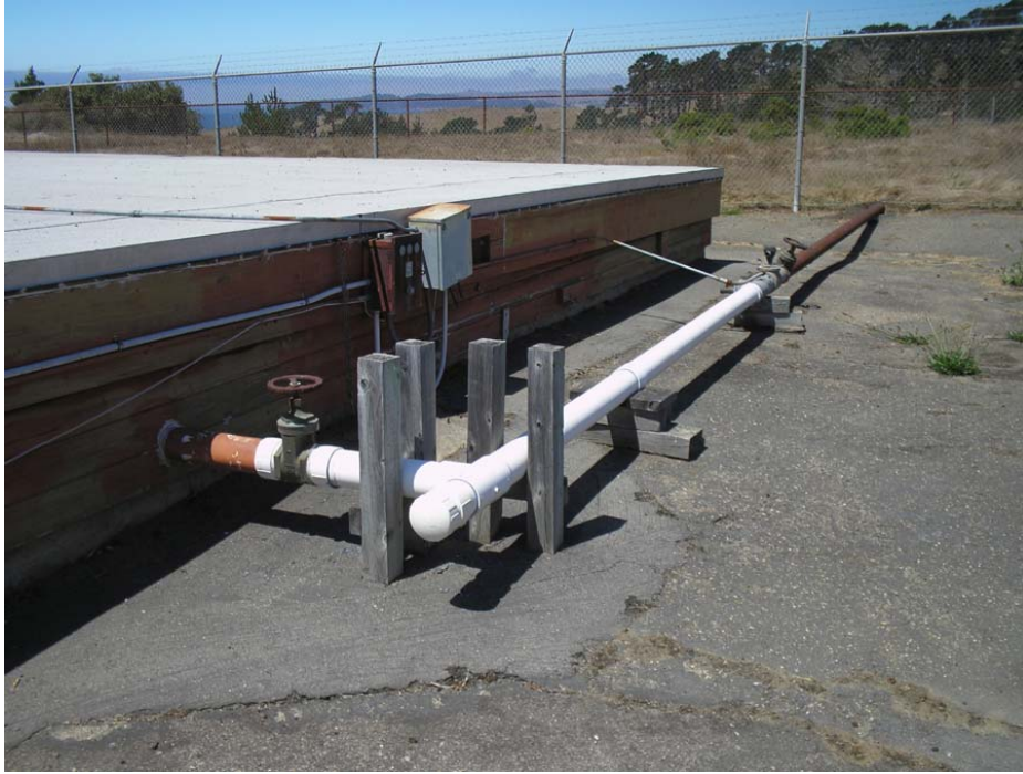
Figure 4-4: Reservoir and Piping
