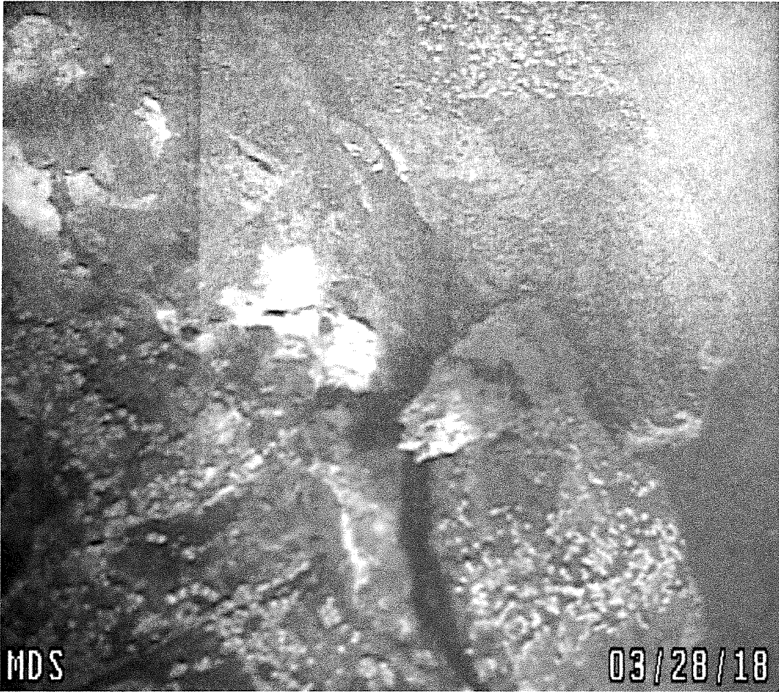
Metal strap is corroded away, corrosion on pipe
