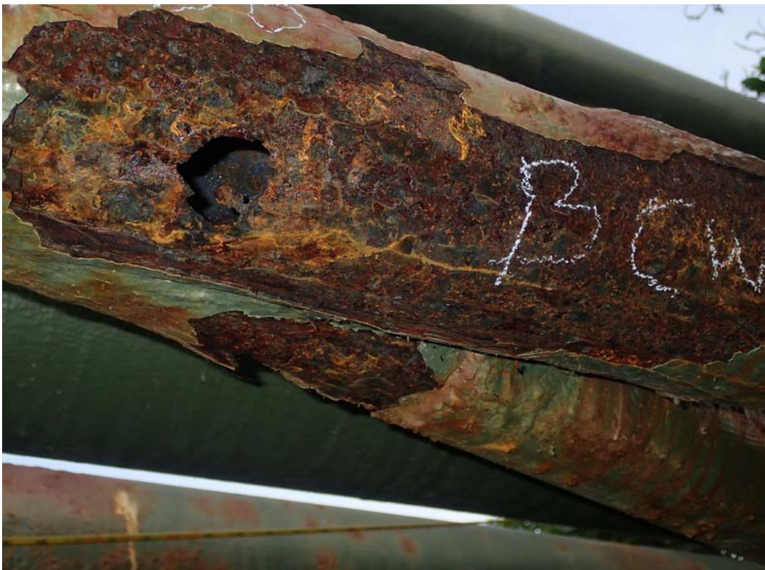
Full thickness corrosion on the bottom chord west side at a connection to a lateral brace.
