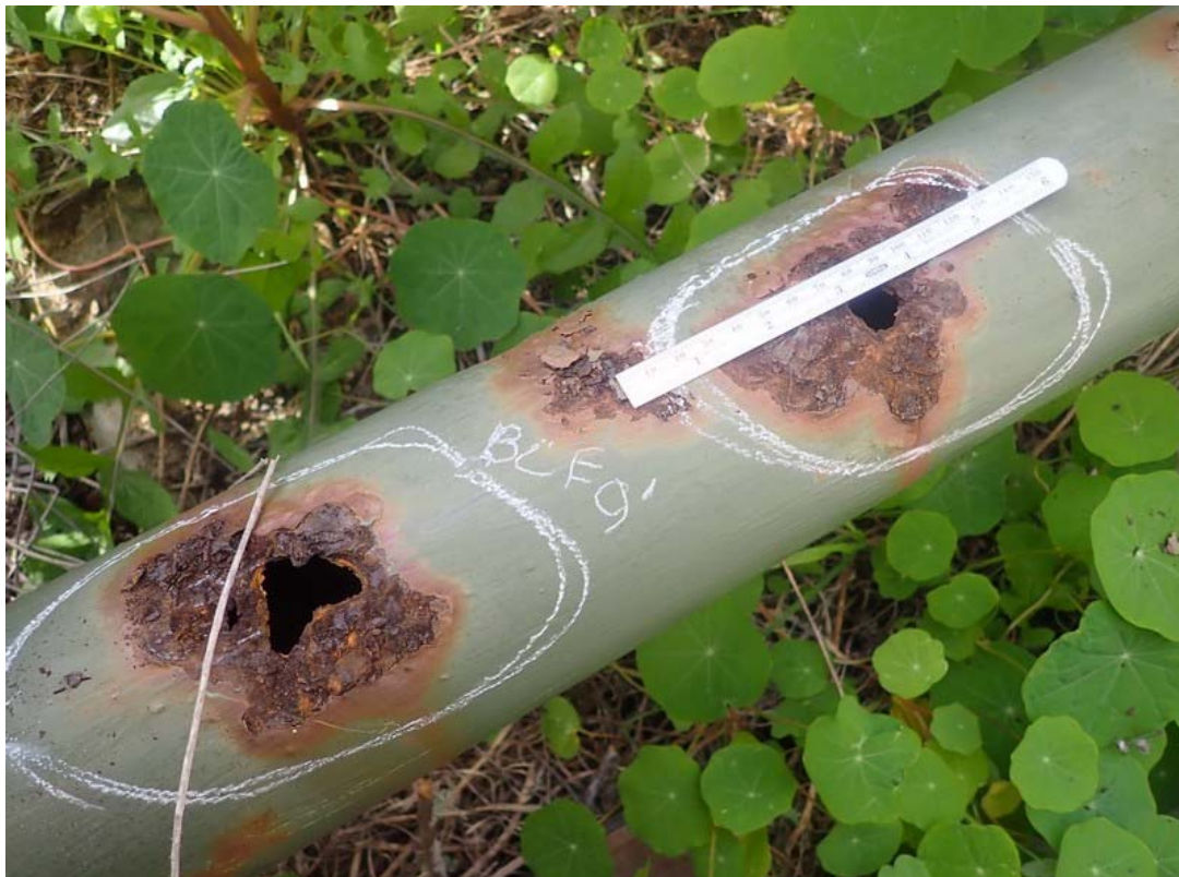
Full thickness corrosion on the eastern bottom chord near the north end.
