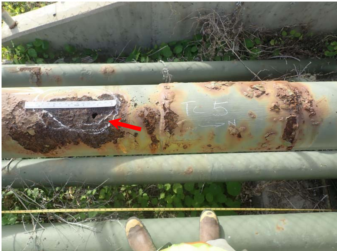
The hole at the arrow is about 5 ft. from the northern end on the top chord. A welded patch from a previous repair is about 6" to the right of the hole.
