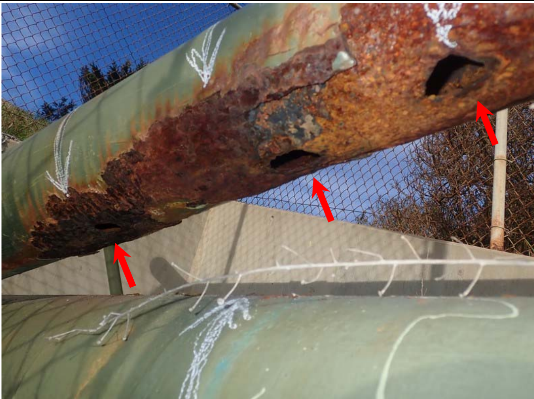
Metal loss is almost complete along the bottom of the vertical brace on the west side 8' from the north end Corrosion is visible on the interior of the holes so there is more damage than can be seen from the exterior.
