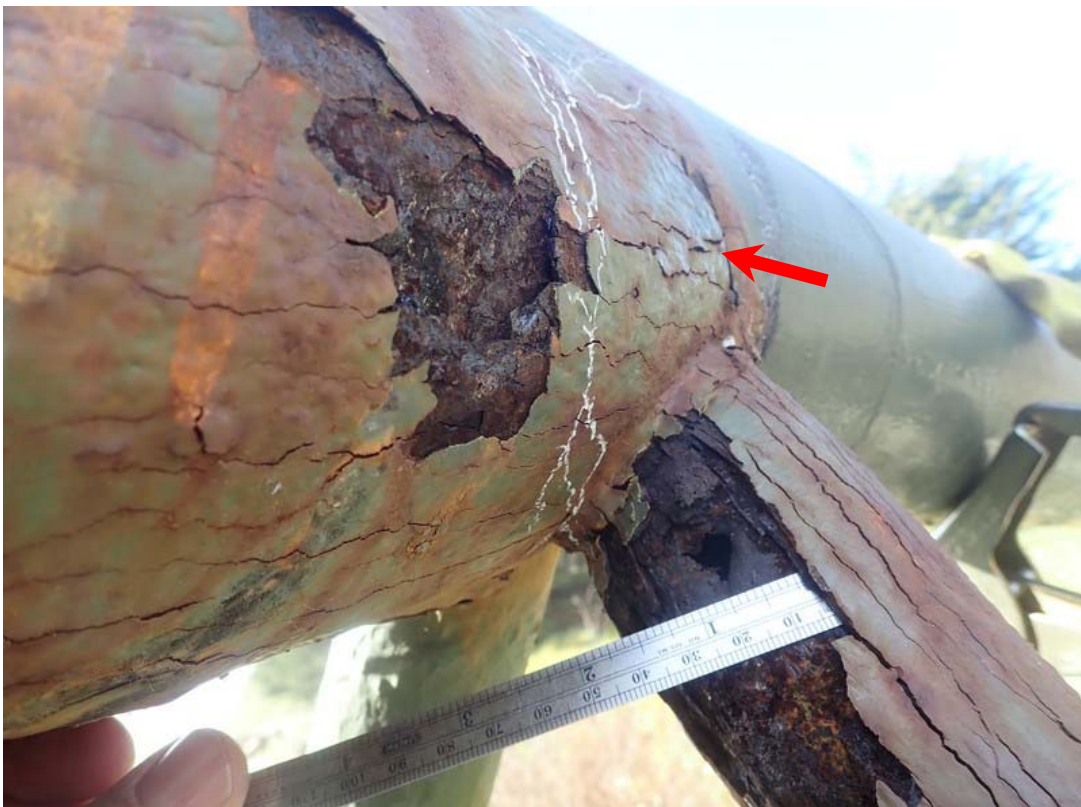
Serious corrosion and metal loss including a hole in the vertical brace. The arrow indicates the top chord.
