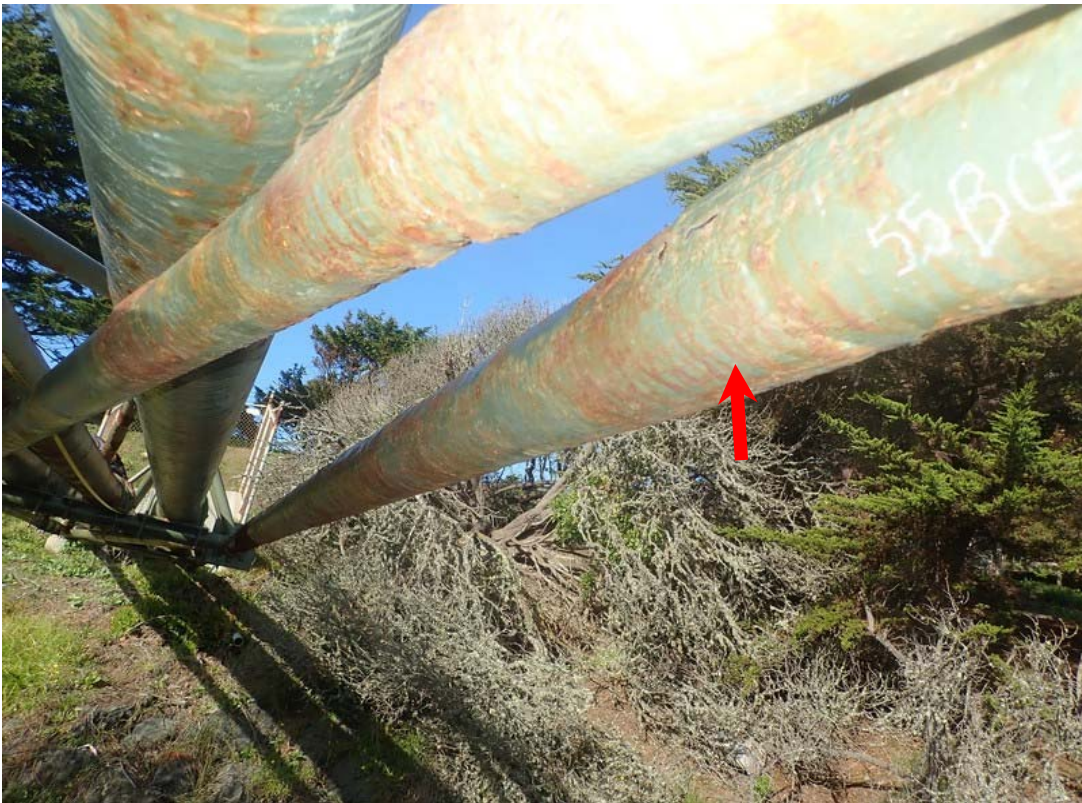
Looking northward on the underside. Coatings have failed and significant corrosion is present under the paint on most surfaces. The arrow indicates the bottom chord which is a primary member.
