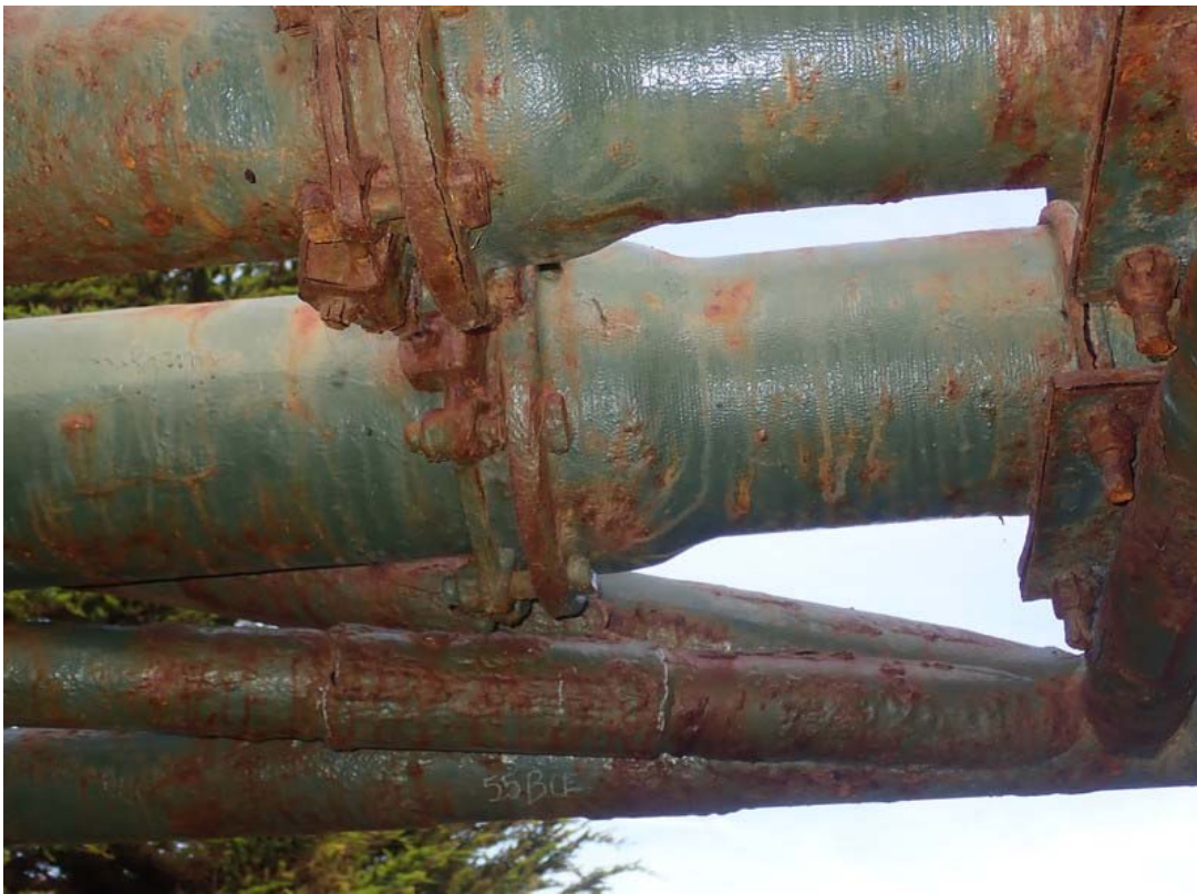
Another view of serious corrosion on the carrier pipes and the bridge from underneath.
