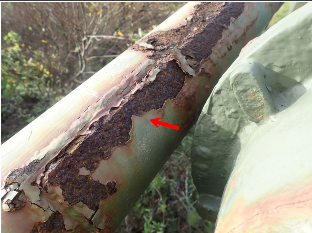
This view shows a welded patch (arrow). The patches are likely from previous repairs of corrosion. Serious corrosion and metal loss surround the patch.
