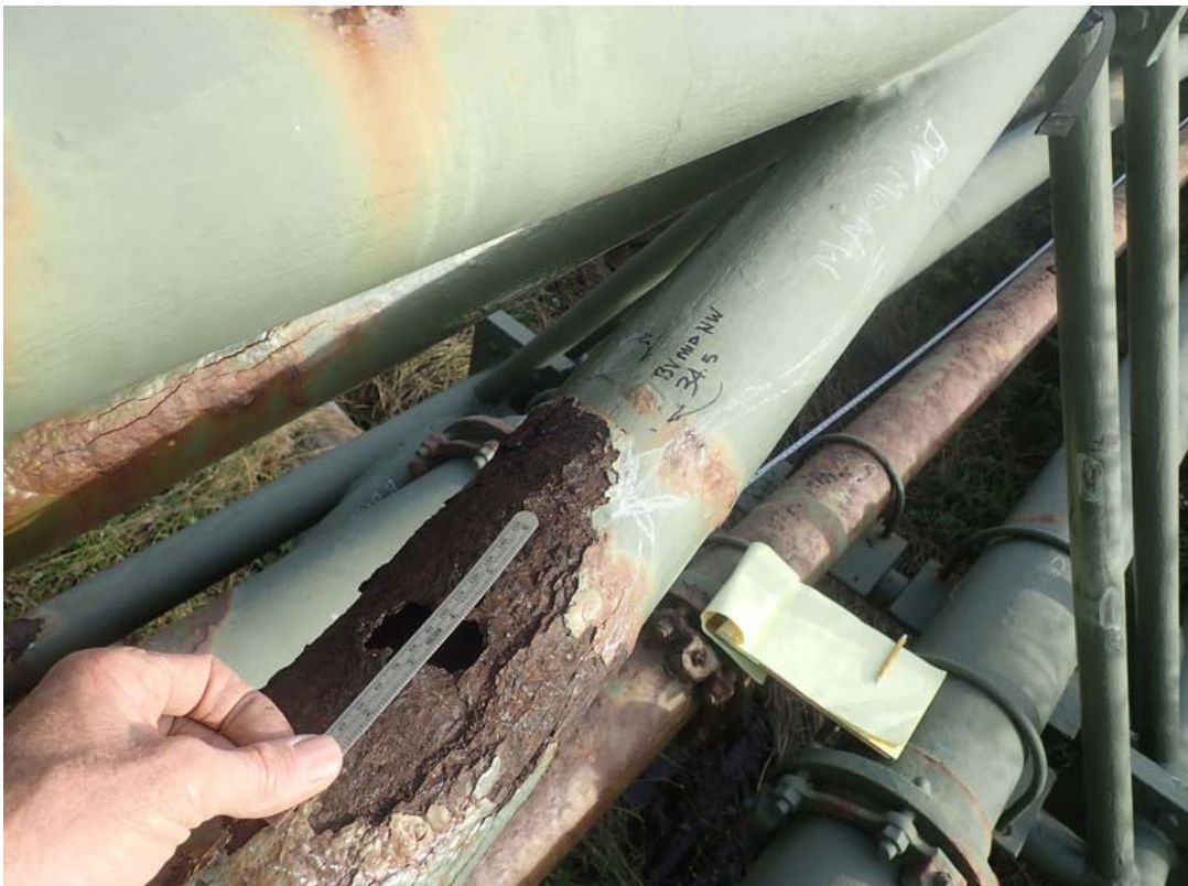
Another example of severe metal loss on this vertical brace on the west side.
