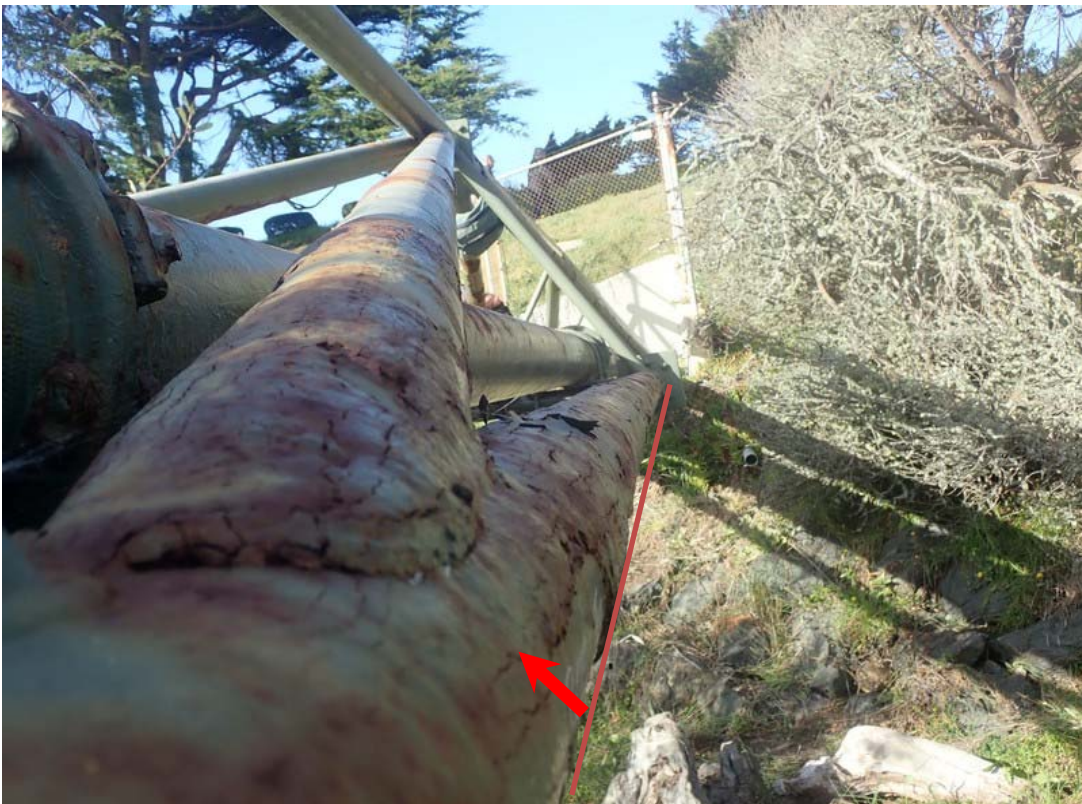
Another view of the eastern bottom chord (arrow) and a diagonal brace. Significant metal loss is present under the lifted coatings. Some deflection (bend) is visible in the member. This could be from original construction or impact.
