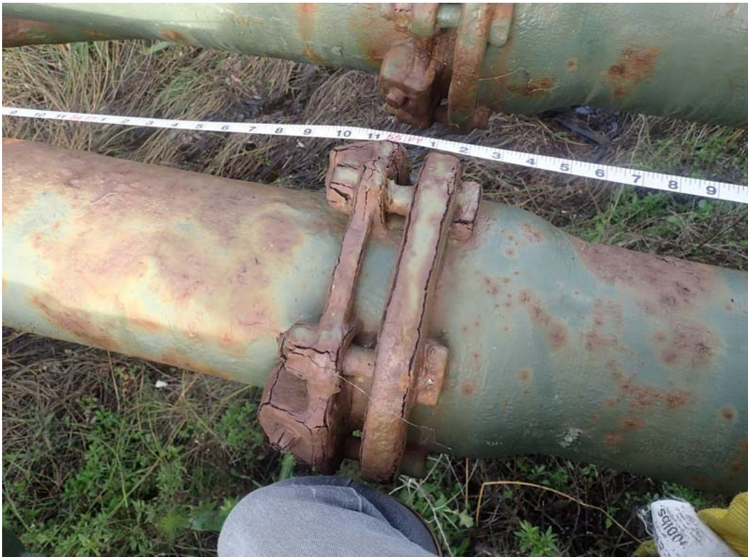
The carrier pipes were not inspected as part of this work but significant corrosion is evident in most areas.
