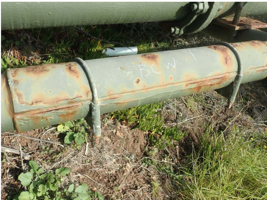
This is a view of the bottom chord on the west side. This appears to be a repair using U-bolts to clamp two "half-pipe" pieces around the original structure. The pieces appear to be caulked to form a non-welded repair. Several of these assemblies are present.
