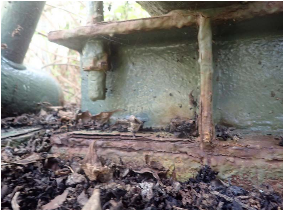
Additional view of corrosion on the southern end at the abutment.
