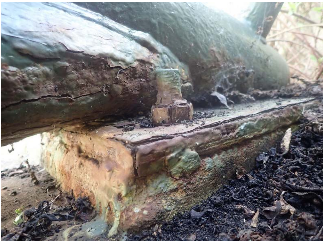
Abutment connection at southern end showing serious corrosion and metal loss on most surfaces.
